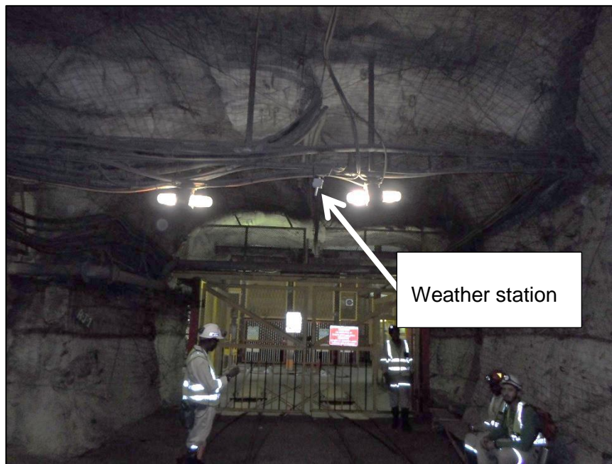
Figure 67: Weather station installed at the 10-level station
