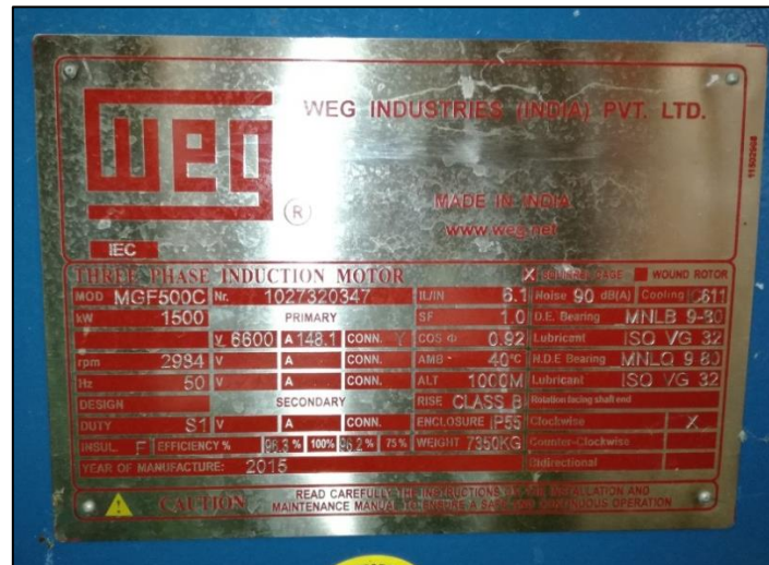
Figure 33: Chiller induction motor specification plate
