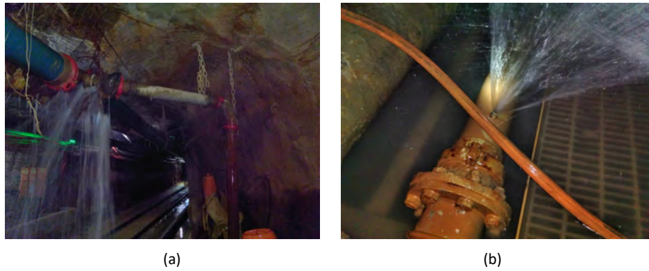
Figure 6.11: Examples of reported water leaks
