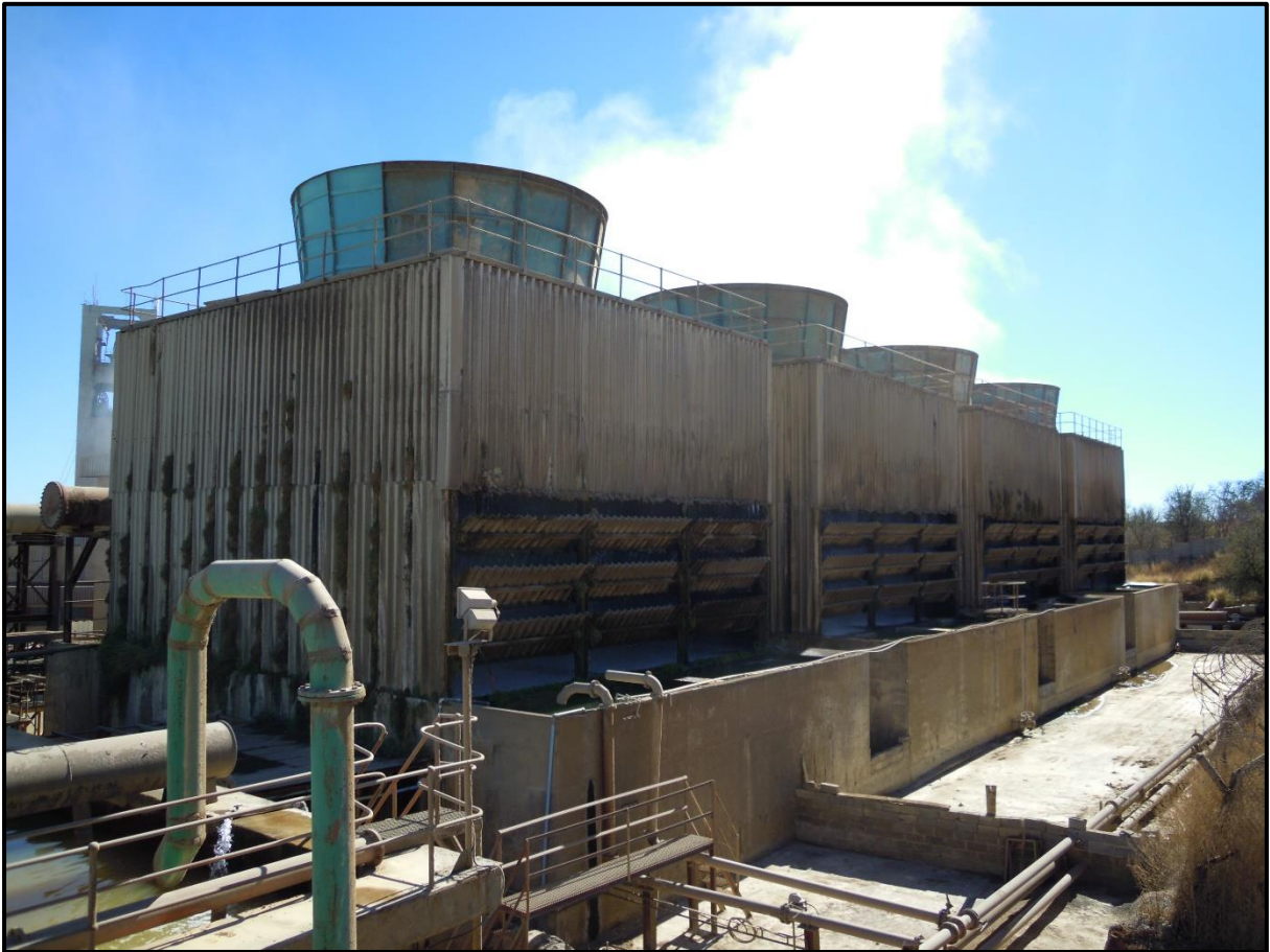
Figure 16: Mechanical draft cooling towers
