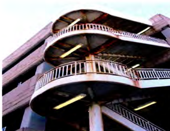
Figure 1.2. Photo showing effect of corrosion
