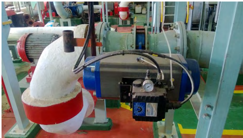
Figure 45: Non-functioning pneumatic control valve
