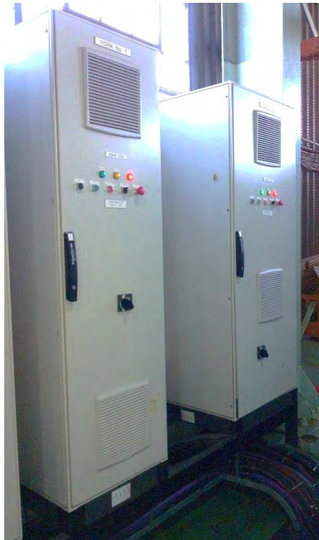
Figure 103: York 4 condenser pump VSD (right)
