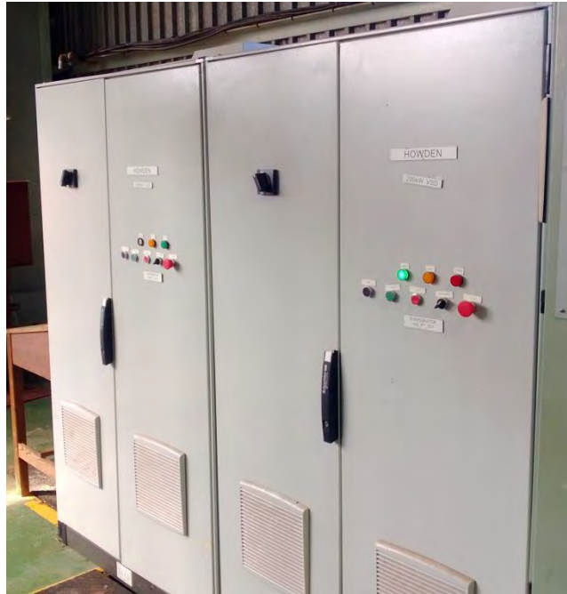
Figure 104: Howden condenser (left) and evaporator (right) pump VSDs
