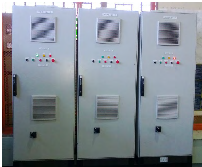
Figure 101: York 1 to 3 condenser pump VSIDS
