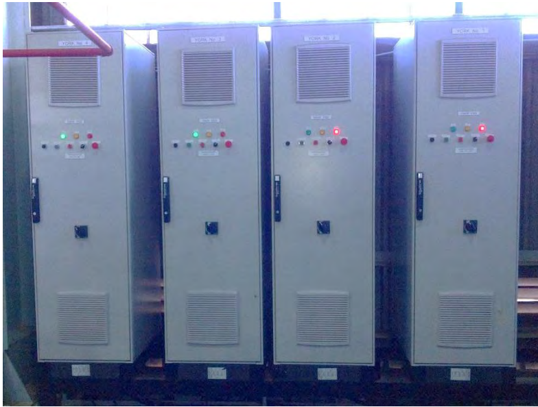
Figure 102: York 1 to 4 evaporator pump VSDS
