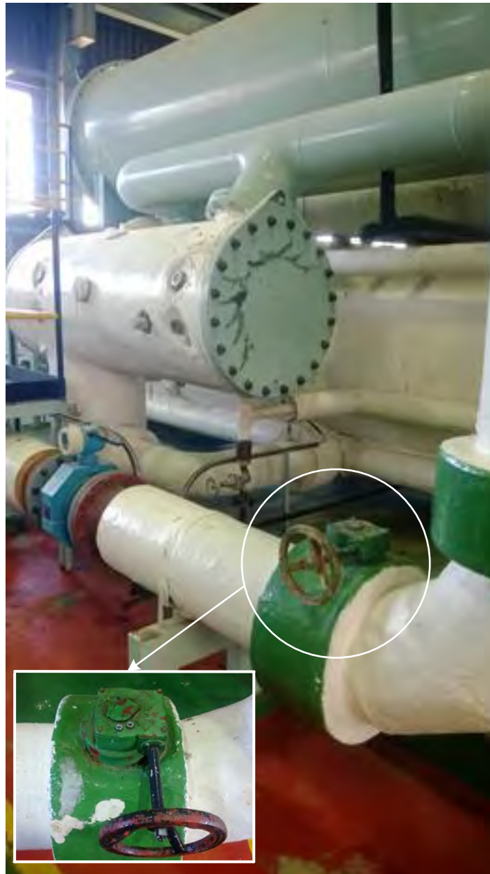
Figure 46: Manual water-flow control valve
