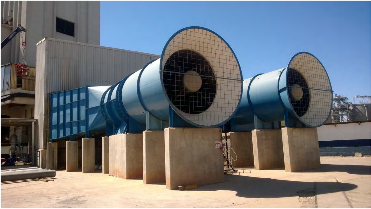
Figure 54: New BAC installed on case-study mine
