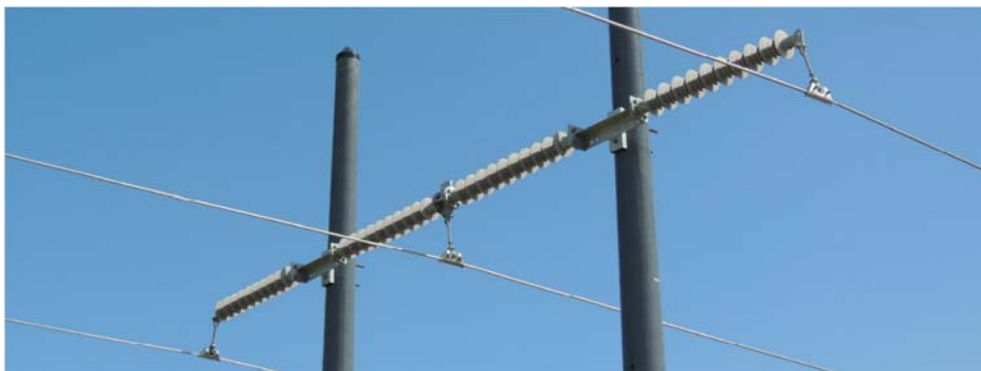
Photograph 1: Insulated cross-arm on H-pole [13]
