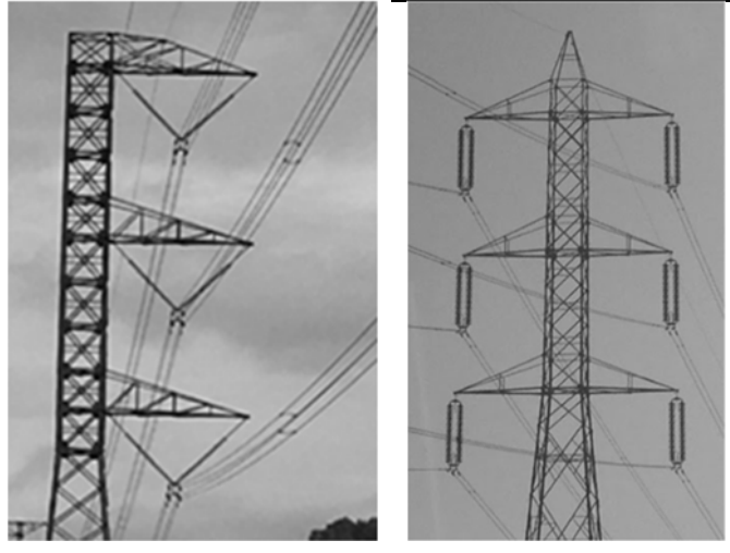
Figure 69: V-Suspension (left photo) and suspension (right photo) insulators
