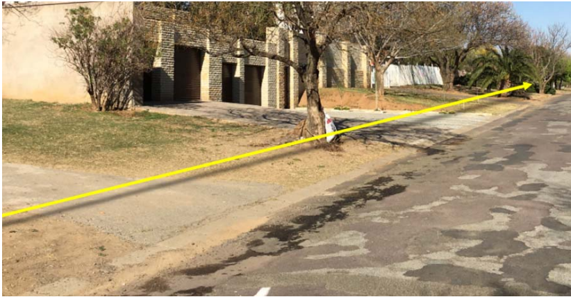
Figure 106: Kroonstad 66 kV Oil-filled cable route overgrown with vegetation
