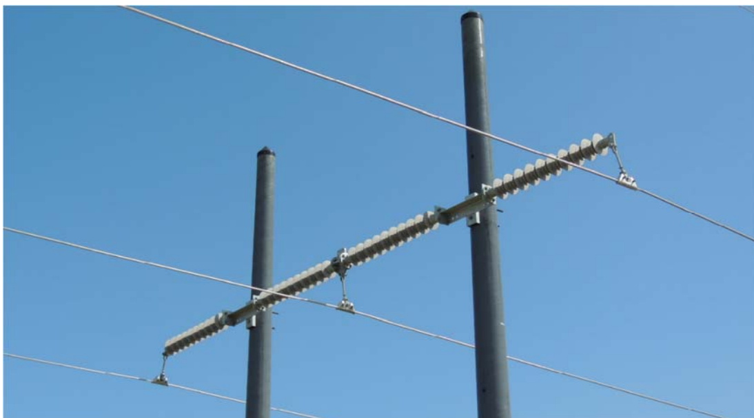
Figure 72: Insulated cross-arm on H-pole [122]
