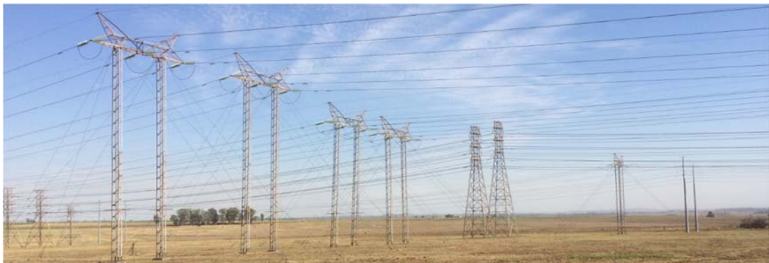
Figure 4: Land use for 88 kV overhead feeder lines
