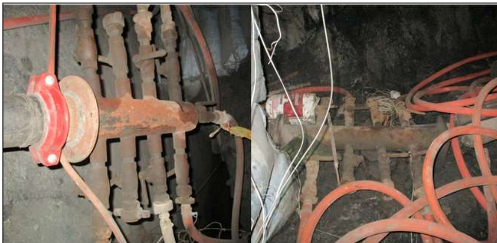
Figure 11: Rubber pipes connected to a compressed air common manifold
