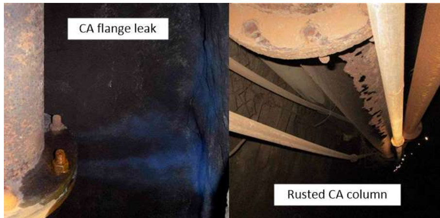
Figure 13: Compressed air flange leak and rusted column
