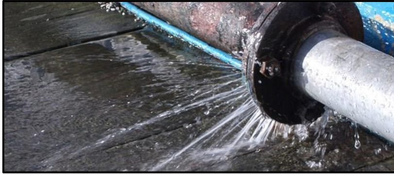
Figure 16: Leaking pipe flange [42]
