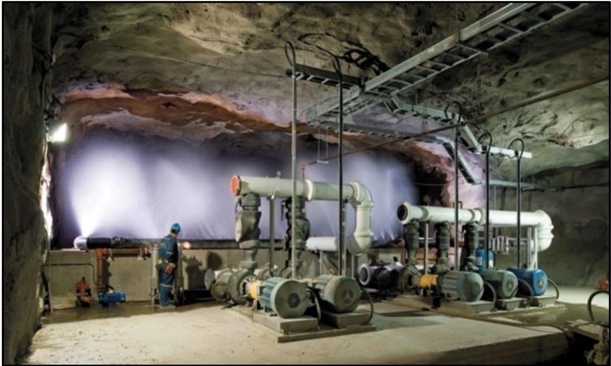
Figure 6: Underground horizontal forced draft BAC with direct-contact spray HX 1
