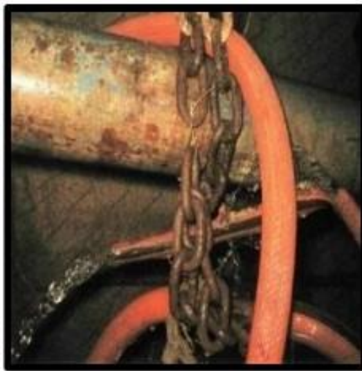
Figure 17: Open chilled-water hose [8]
