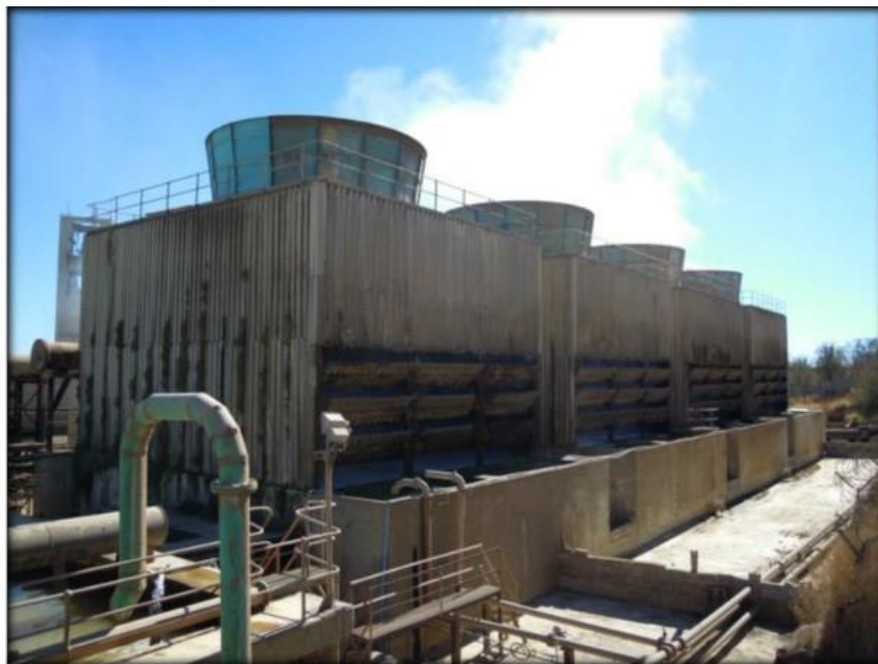
Figure 15: Practical example of pre-cooling towers [34]
