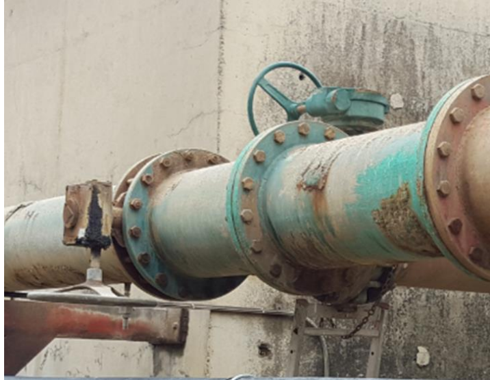
Figure 46 - Actuated valve installation
