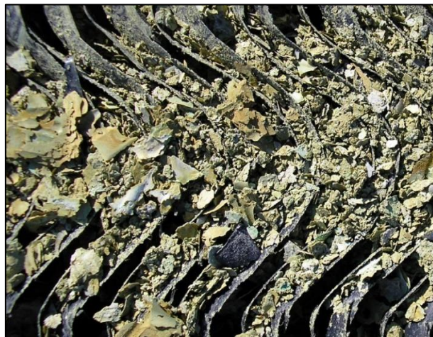
Figure 20 - Severe scaling on fill [25]
