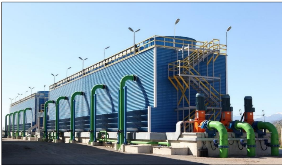
Figure 15 - Cooling tower example
