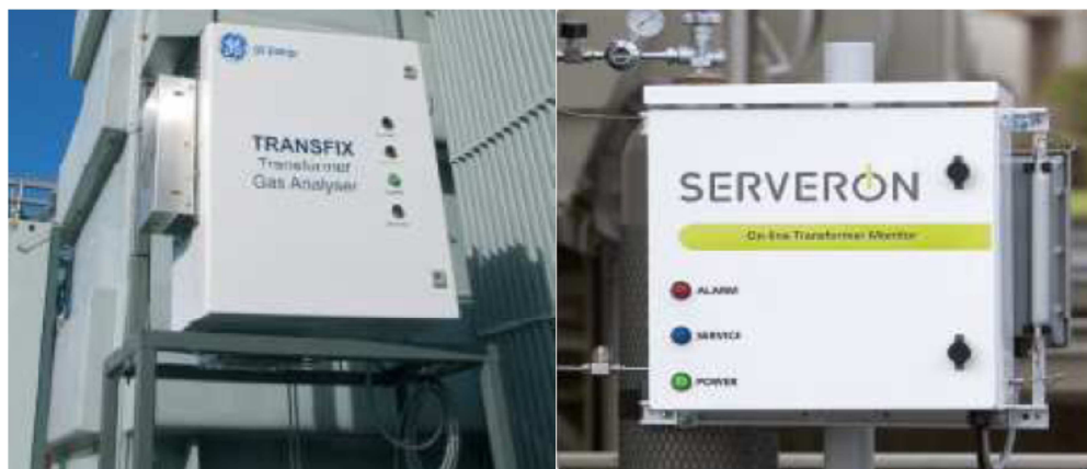
Figure 2-8: Two makes of gas analysers used in Eskom Transmission
