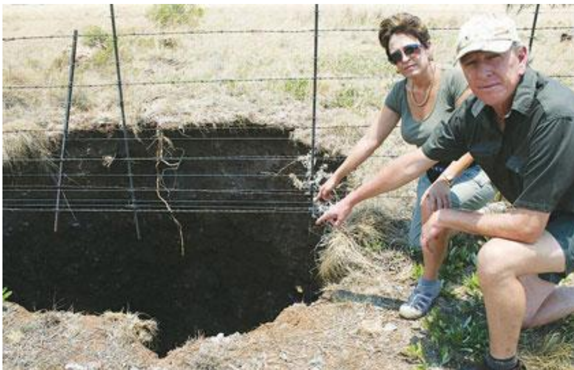
Photo 4-2: Land owner pointing out a sinkhole that formed on the extended pipeline
