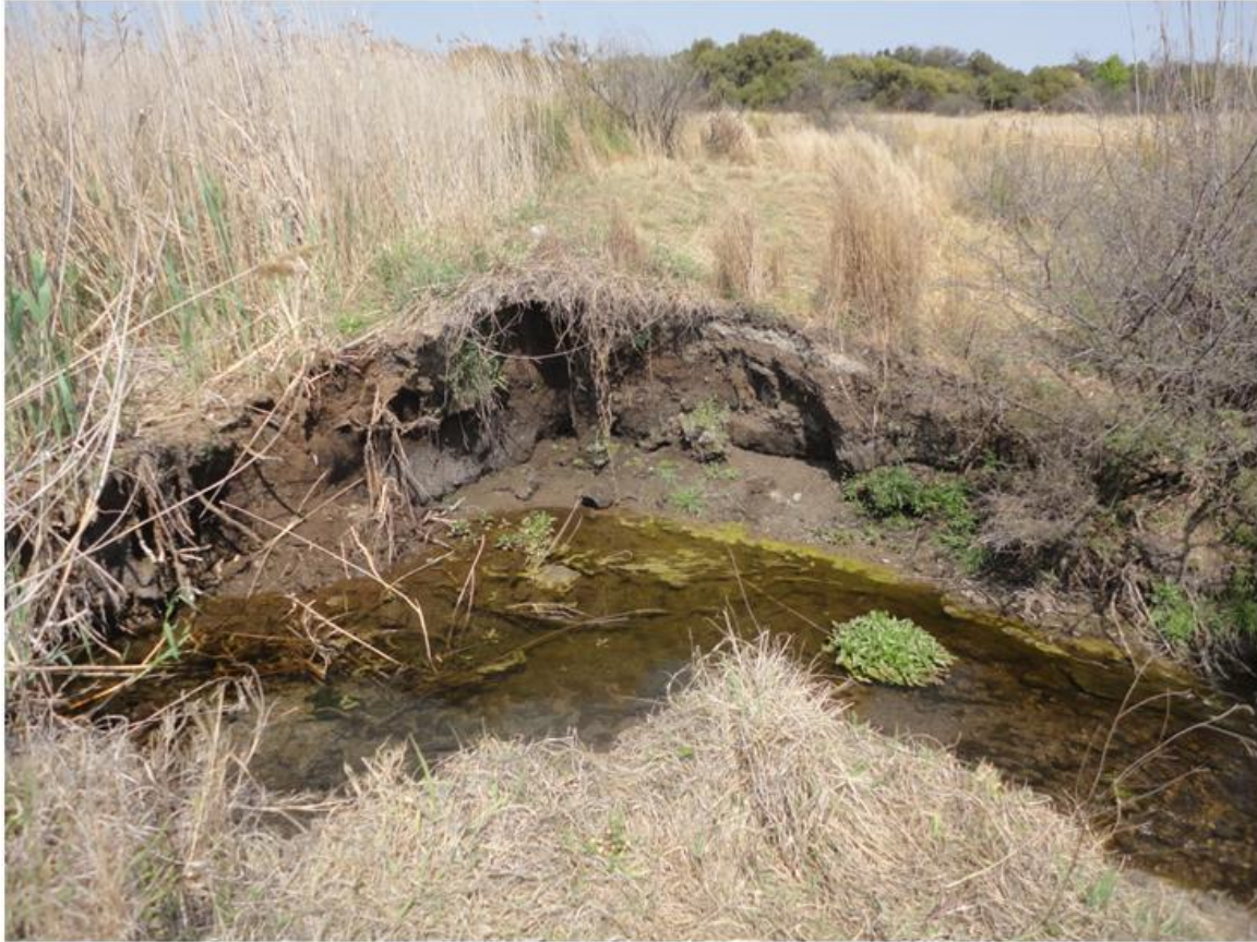
Photo 4-1: Breached retention wall at Rietpoort Spring
