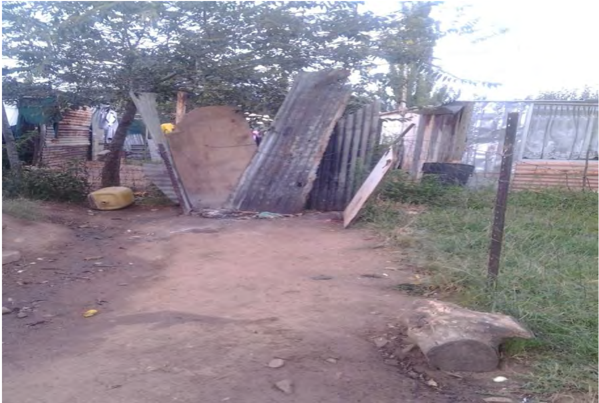
Photo 27: Pit latrine that has collapsed due to uncompleted construction (Source: M. Mokoena, 2015)
