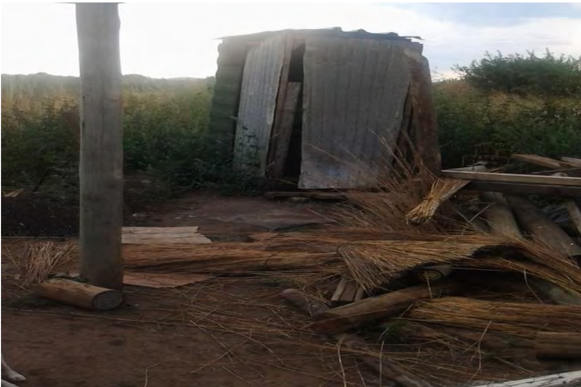
Photo 24: An unstable pit latrine (Source: M. Mokoena, 2015)
