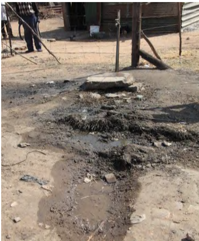
Photo 19: Damp, poor drainage and stagnant water at one of the communal taps (Source: M. Mokoena, 2015)
