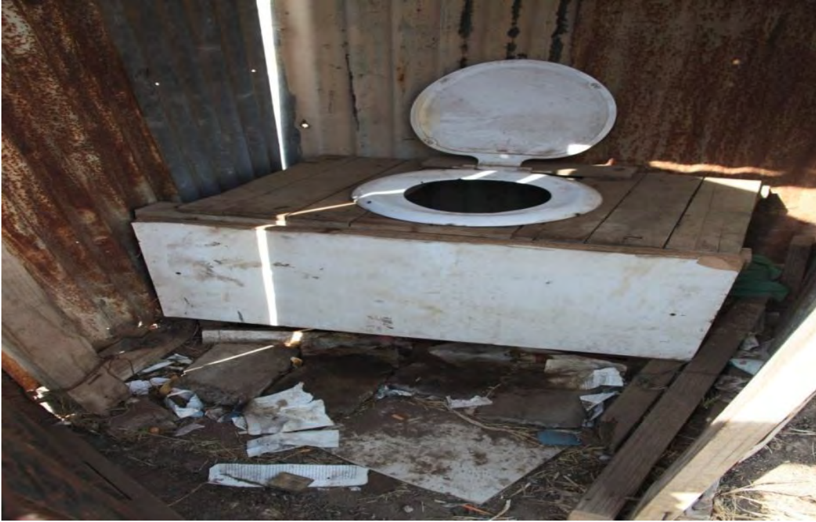
Photo 23: Dirty and unhygienic latrine in BIS (Source: J.W.N. Tempelhoff, 2015)
